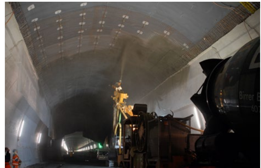
Fig 2.6: Installation of a tunnel ceiling with variable shape by means of sprayed concrete onto membrane with the help of wire mesh (walls have been built with formwork and in-situ concrete)
