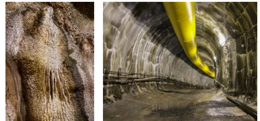
Fig 3.2: Damage due to insufficiently durable shotcrete (e.g. crystallization pressure due to sulphate attack)
